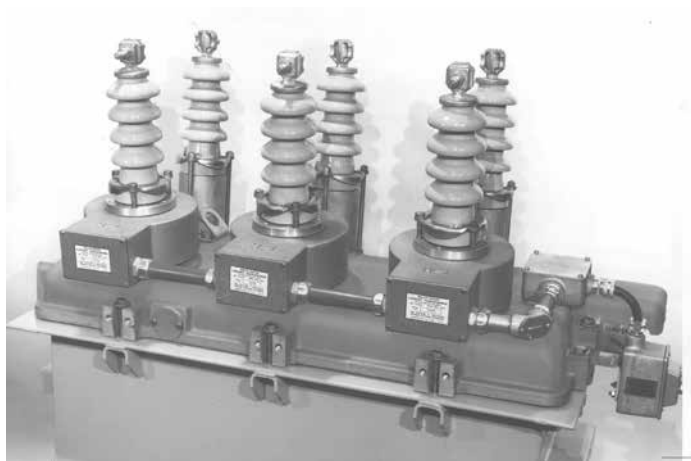
Figure 11. Multi-ratio current transformers mounted on the source-side bushings.
