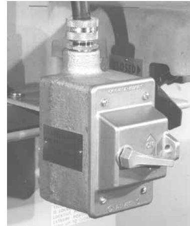
Figure 15. Ground-trip blocking switch for remote manual operation.
